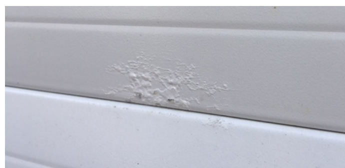
Salt corrosion caused by salt trapped between slats.
