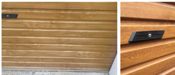
Fading due to weathering / UV radiation over time - left image compared to image of new door (right).
