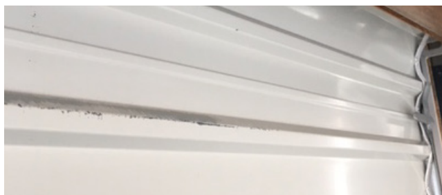
The above image shows normal wear & tear to the inside of the roller door curtain.
